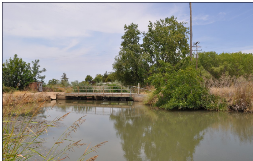
El Nido Dam on Mariposa Creek will be automated, helping El Nido area growers to maximize water rights from Mariposa Creek during times with high flow.
