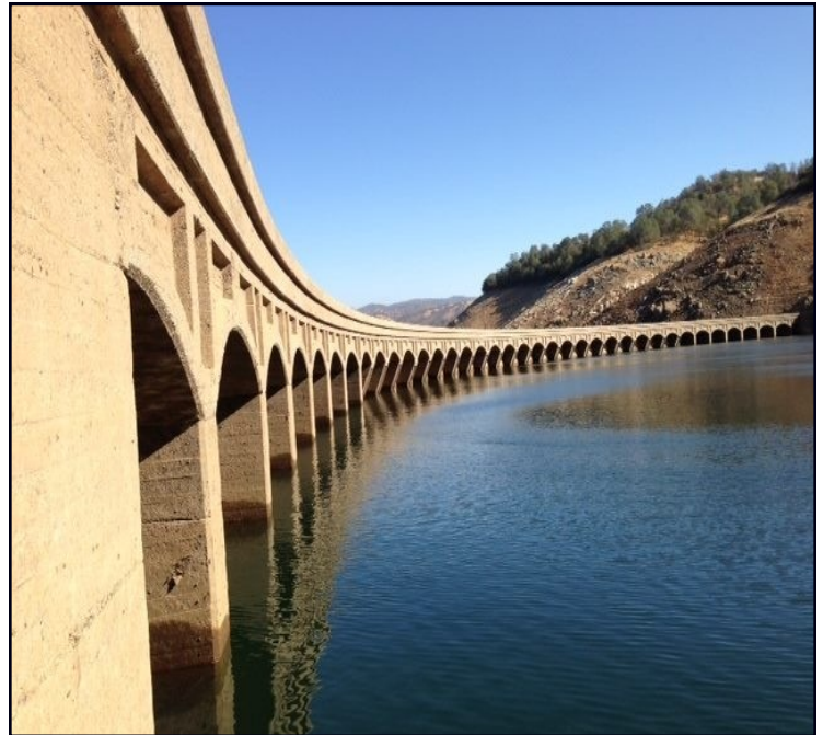
The original Exchequer Dam continues to emerge from Lake McClure as the water level drops in a second dry year. This is the top of the original 1920s dam as seen in early November.
